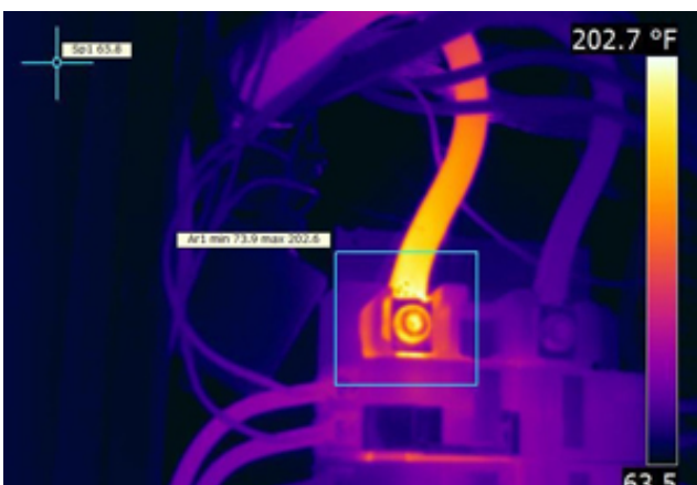
An overloaded cable or a poor connection
